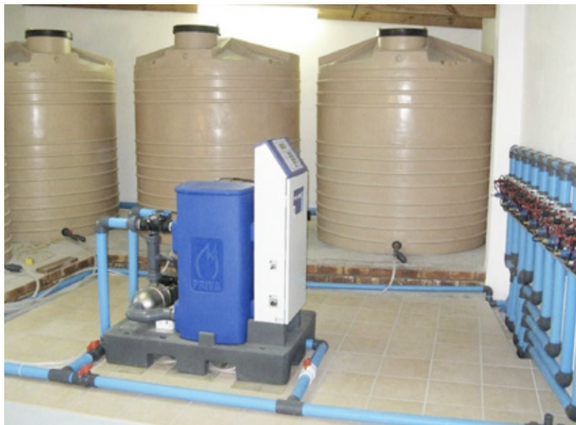
Irrigation pump room showing fertigation tanks and fertigation dosimeter
