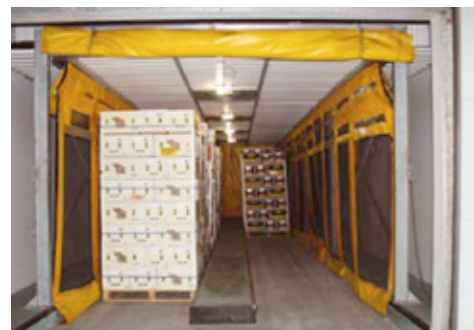
Forced air cooling tunnel
